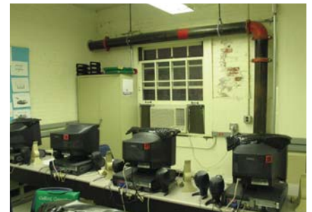
Basement Level Computer Room at Adams Middle School
